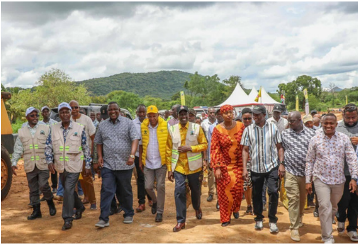
Principal Secretary Eng. Joseph Mbugua, alongside national and local leaders, accompanied H.E. President William Ruto on an inspection tour of the 55km Mto Mwangodi–Dawida–Mbale–Wundanyi–Bura Junction Road in Mwatate Constituency, Taita Taveta County, on 10th April 2026.
