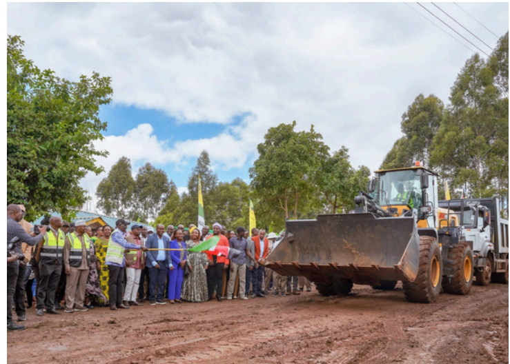
H.E. President William Ruto presides over the launch of construction works for the Kiriko–Kagumoini–Gitugi–Chui–Karugia Road (RWC 690) in Murang'a County on 24th April 2026.
