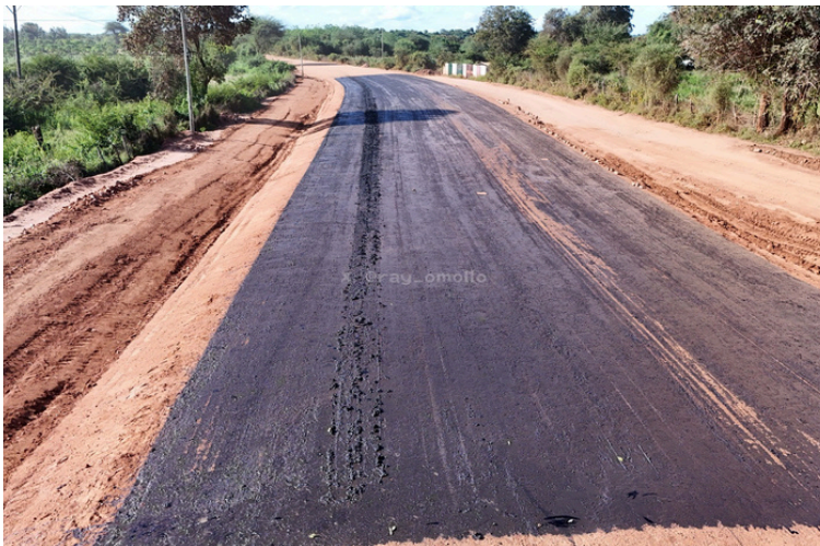
Construction works ongoing on the 13-kilometre Kamuwongo–Kandwia Road being upgraded to bitumen standard in Kitui County.
