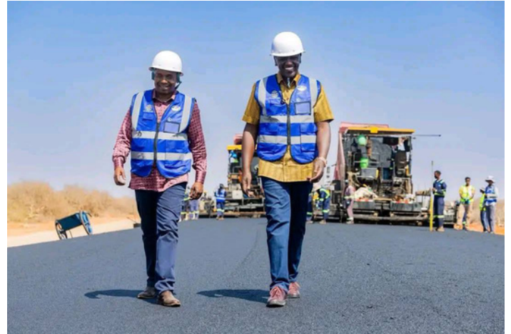
President William Ruto (right), alongside his Deputy Kithure Kindiki, inspects a section of the Isiolo–Mandera Transport Corridor in February, 2026.
