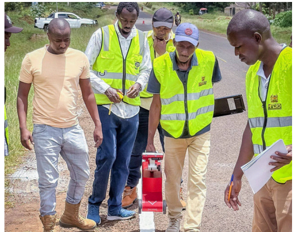
MTRD team leads road marking along the Chiakariga-Meru (B65) Road in collaboration with KenNHA on 20 th April, 2026.
