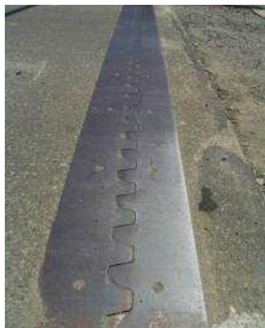
Abnormal clearance of expansion device (no gap)
