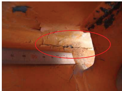
Crack at the upper end of the main girder web
