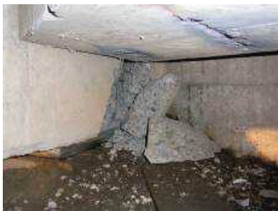
Collision between the girder and the backwall
