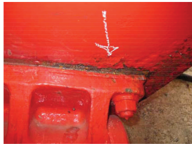
Cracking of paint film on sole plate
