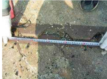
Deviation of expansion joint
