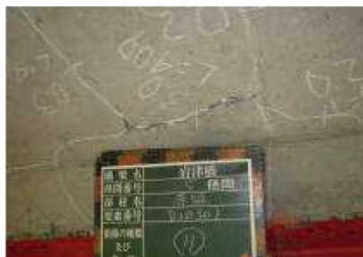
Cracks with falling edges
