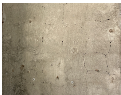
Floor cracks (Bi-directional)
