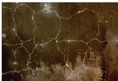
Cracks (floor slab bridges)
