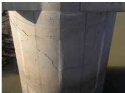
Cracks in the column (shear cracks)
