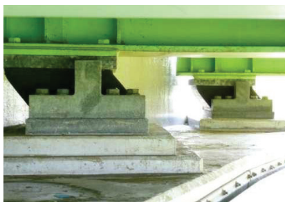
Residual horizontal displacement of rubber bearing
