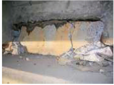
Damage to concrete edge of the cross girder
