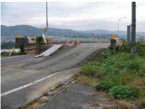
Level difference on the road surface behind the abutment
