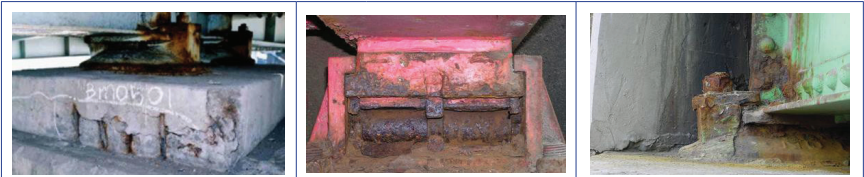
Damage to bearing seat mortar Corrosion of bearing Abnormal movement
