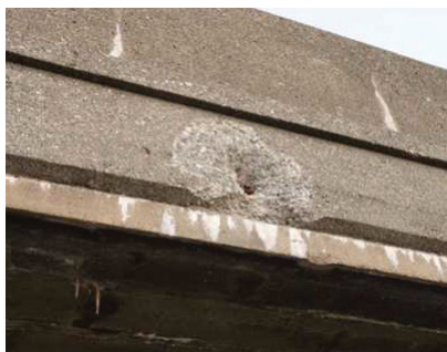
Damage to the fixing section
