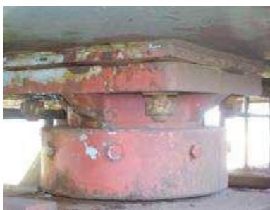
Loose set bolt
