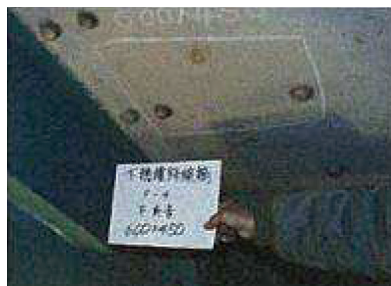
Loosing of steel sheet adhesion
