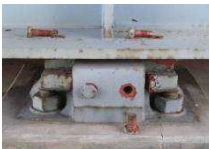
Breakage of set bolt/side block mounting bolt
