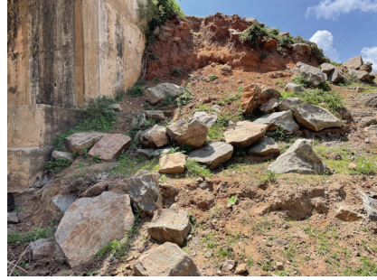
Sediment runoff from side of retaining wall
