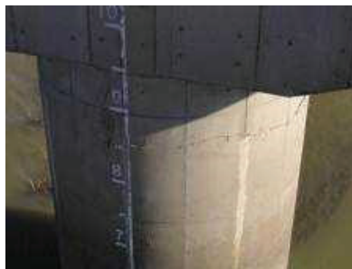
Crack in the column
