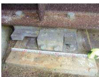
Abnormal clearance of movable bearing
