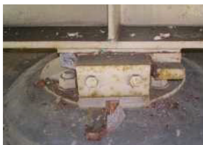
Upper shoe stopper rupture
