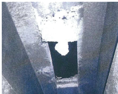
Drop-out of filling concrete
