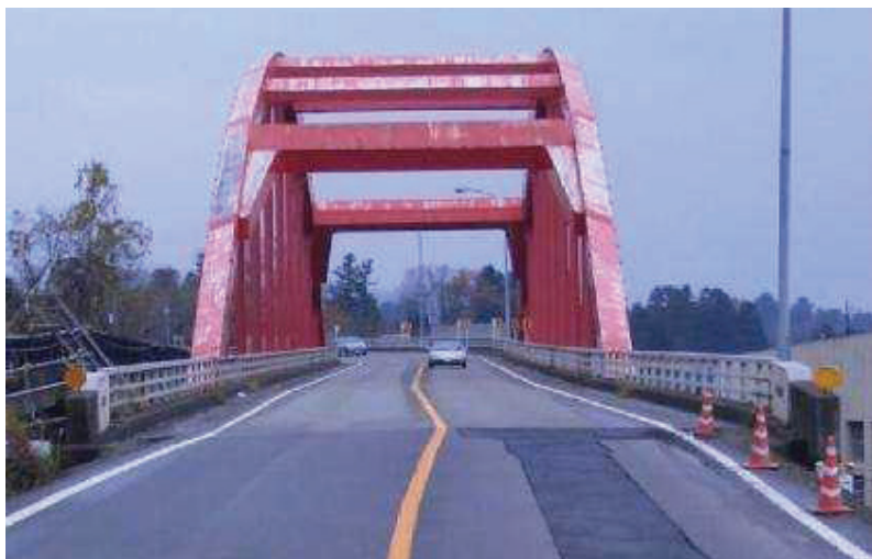
Linear deviation (when there is excessive residual displacement/ foundation movement)
