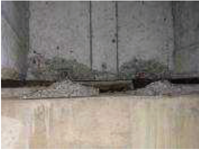
Damage to concrete on the end lateral girder
