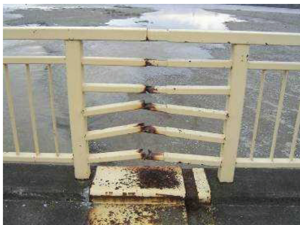
Breakage of the telescopic section
