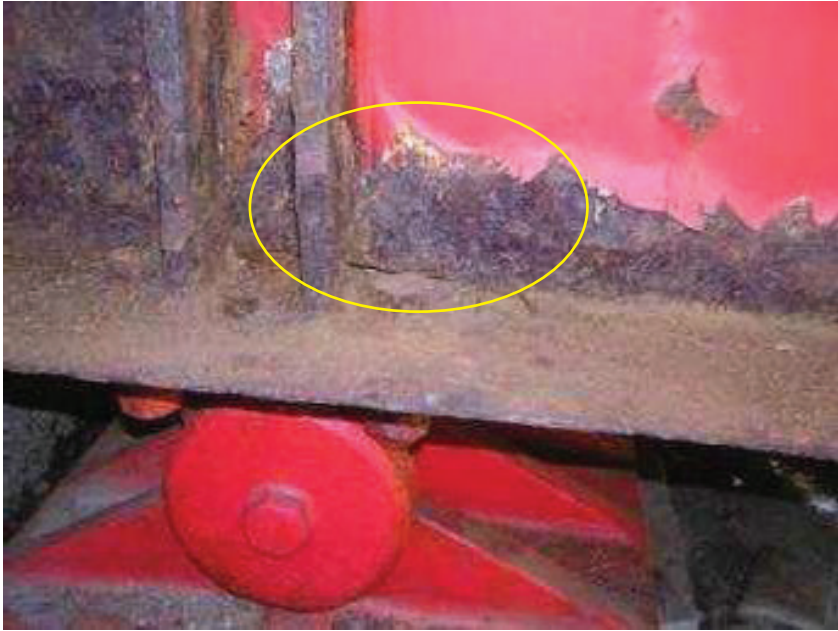
Defective web due to corrosion wall thickness, effect on other parts and the need for immediate repair.
