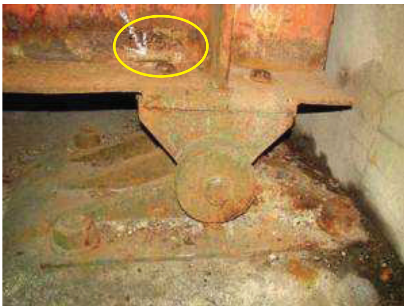
Influence of corrosion wall thickness loss on other parts,
