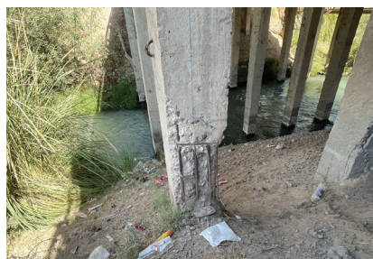
Peeling/Reinforcing Bar Exposure
