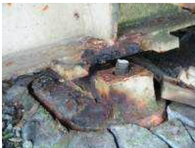
Settlement and anchor bolt rupture
