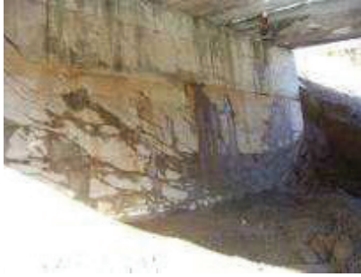
Damage to the vertical wall
