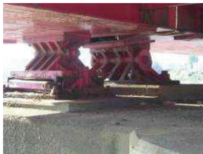
Deformation of the lower flange
