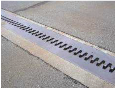
Level difference of the expansion joint
