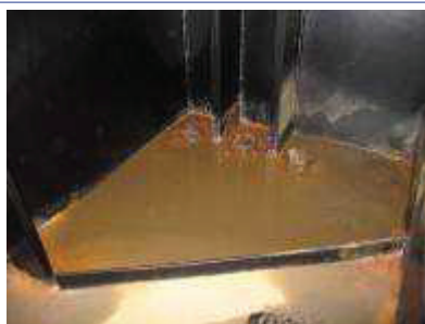
Stagnant water inside the box girder
