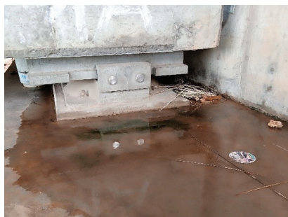
Stagnant water on the bearing seat area
