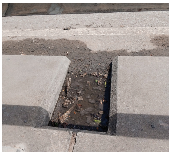
Clogged drainage system
