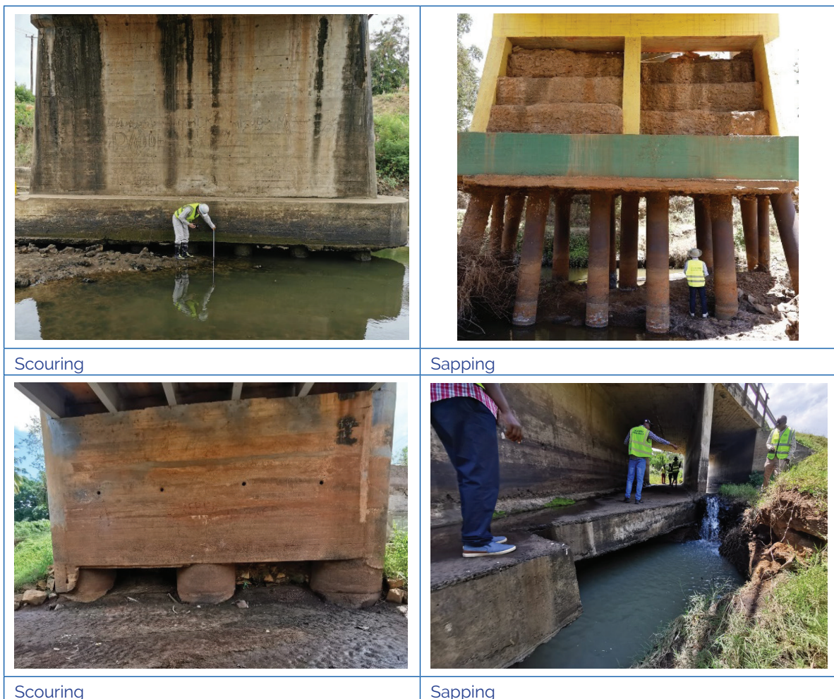
Figure 3.65 Sample photos of foundation deterioration
