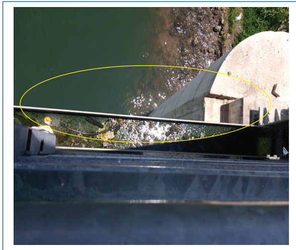
Figure 3.40 Sample photo of water accumulation
