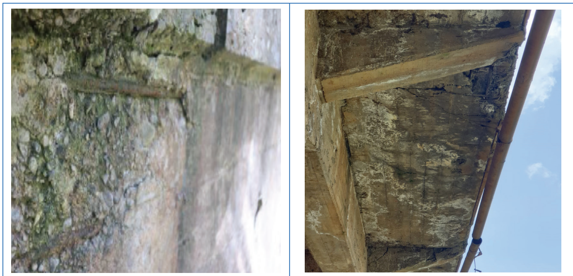
Figure 3.12 Sample photos of carbonation
