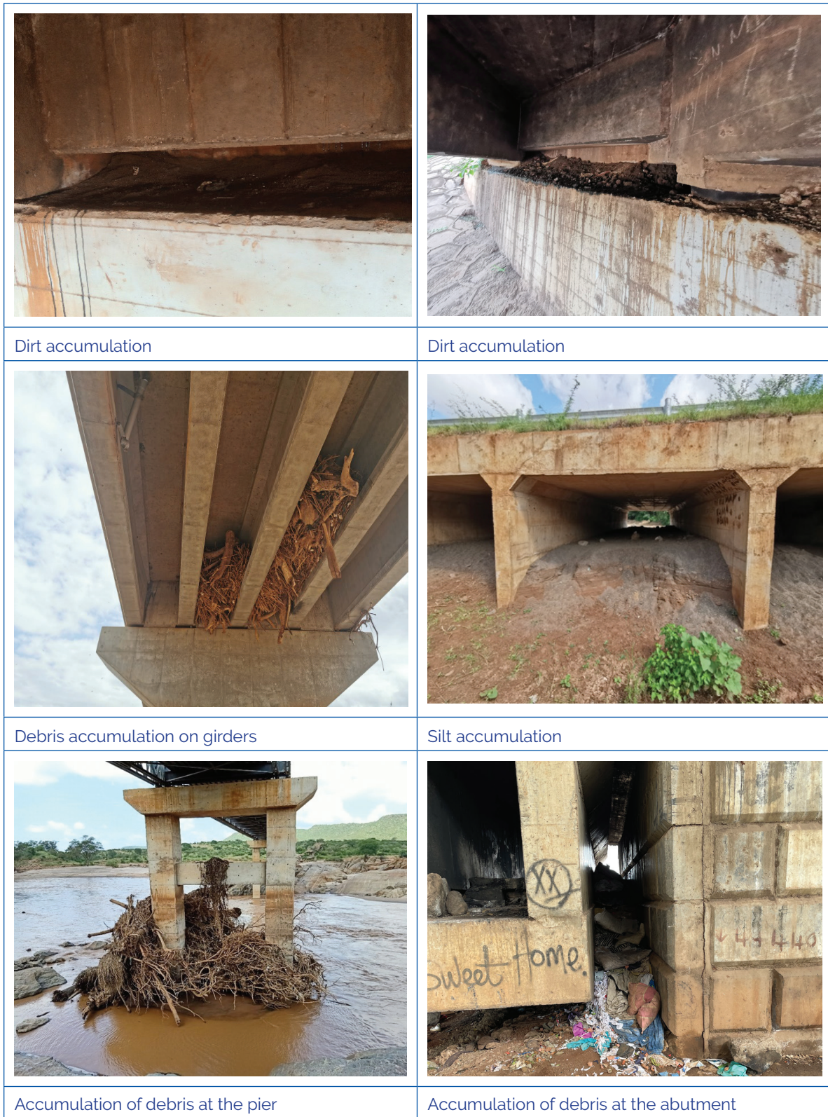
Figure 3.1 Sample photos of siltation on bridge components
