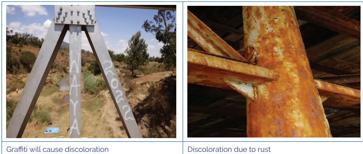
Figure 3.41 Sample photos of discoloration
