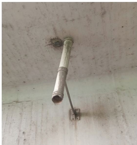
Broken drainage system
