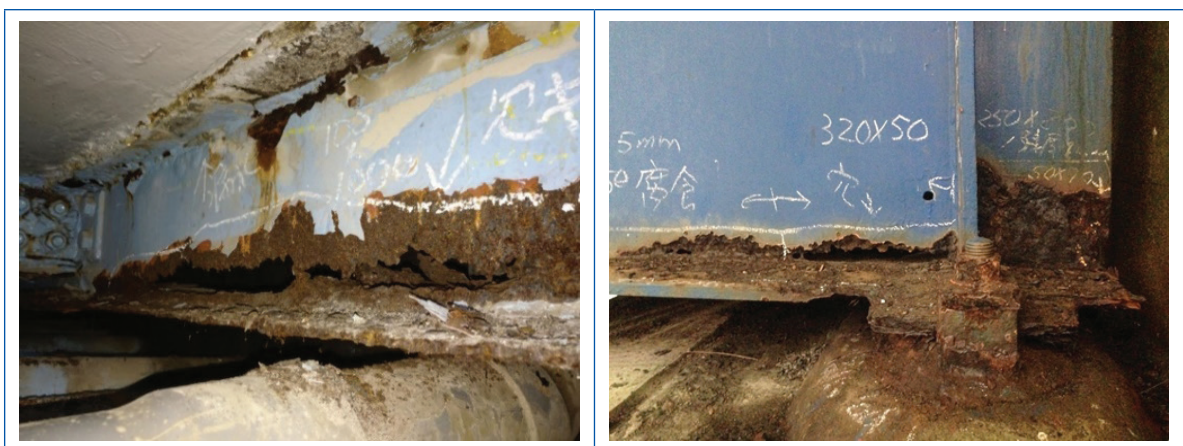
Figure 3.32 Sample photos of section loss caused by corrosion.
