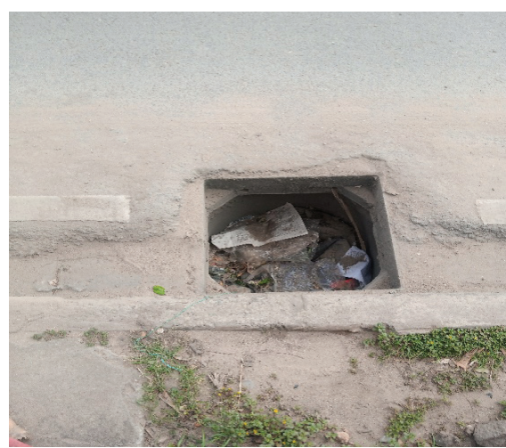
Missing manhole cover
