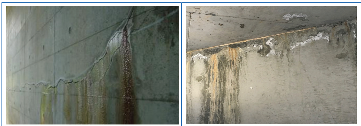
Figure 3.18 Sample photos of leaching and staining
