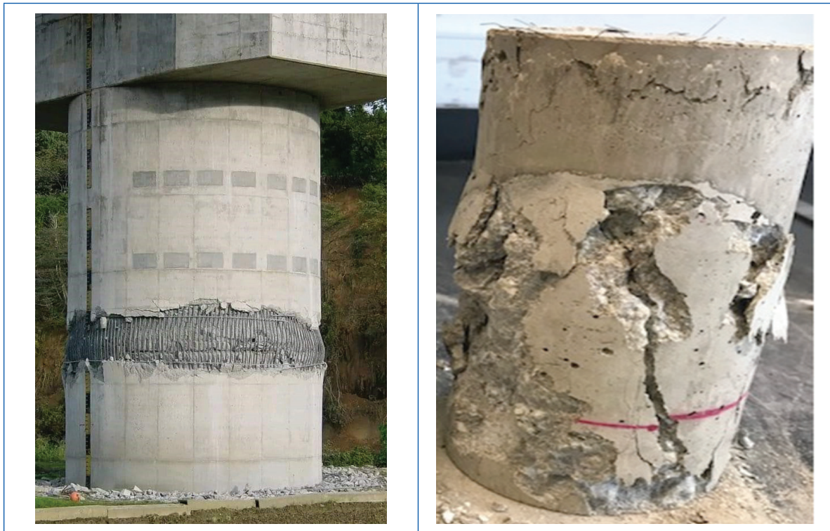
Figure 3.23 Sample photos of buckling
