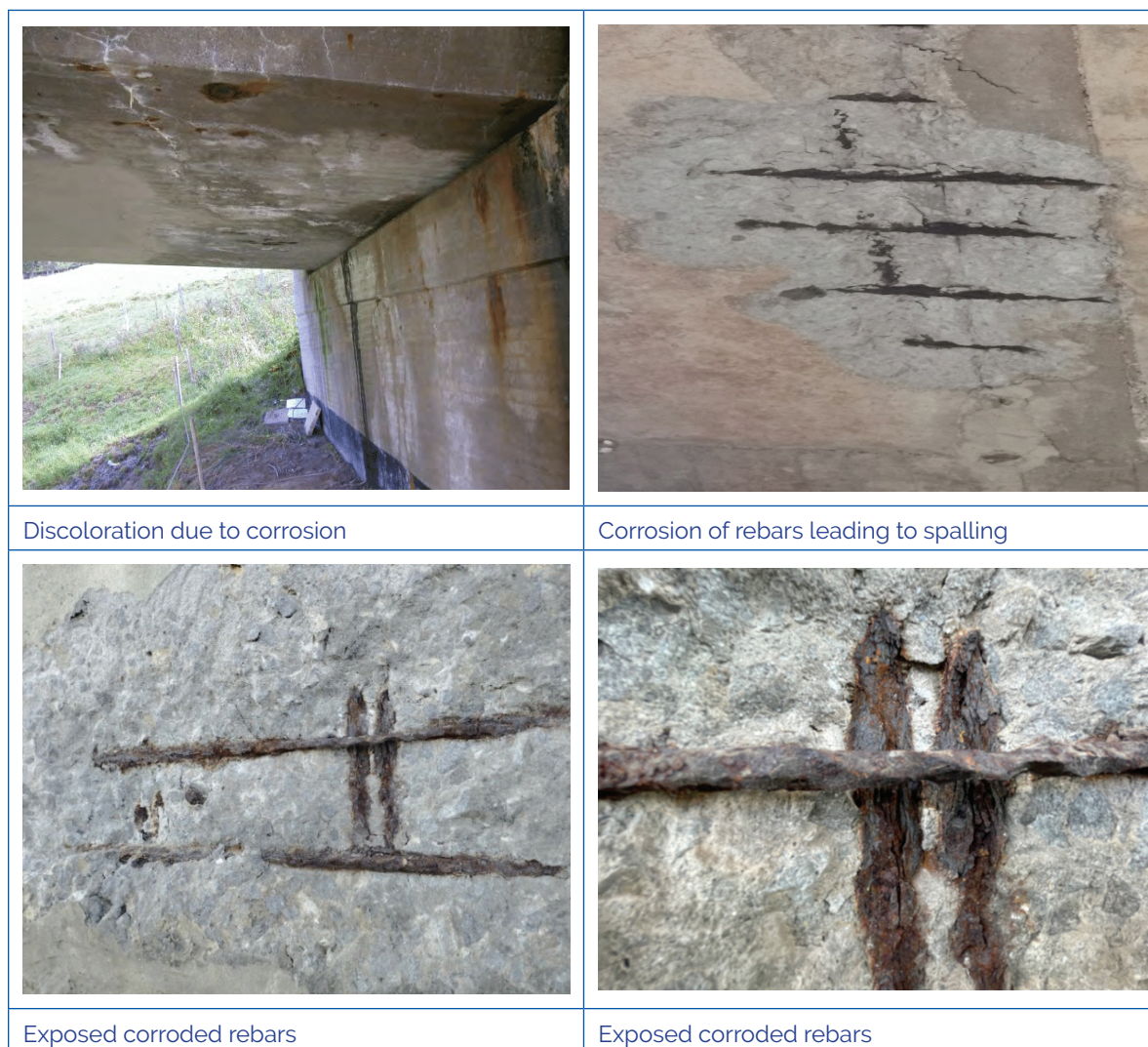
Figure 3.2 Sample photos of corroded rebars
