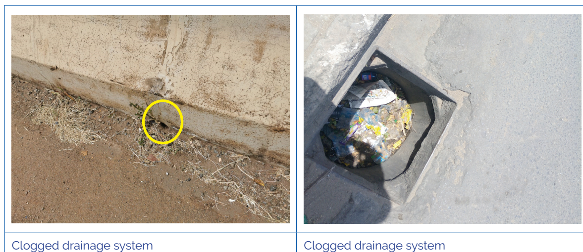
Figure 3.59 Sample photos of drainage system deteriorations
