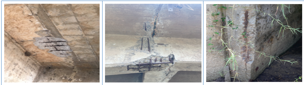
Figure 3.7 Sample photos of rebar exposure/corrosion
