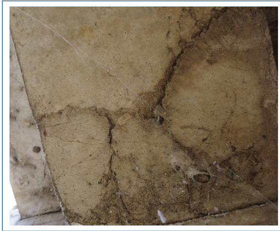
Figure 3.9 Sample photos of delamination
