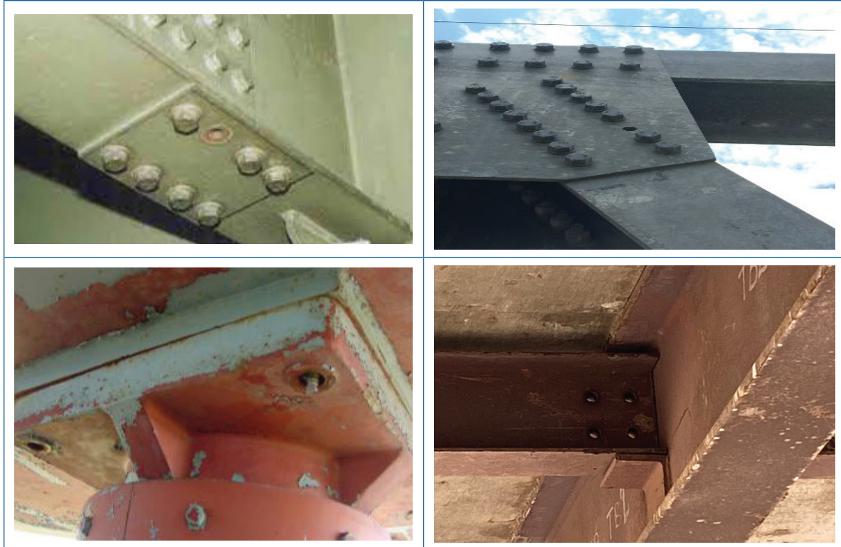
Figure 3.39 Sample photos of loose connection/missing bolts
