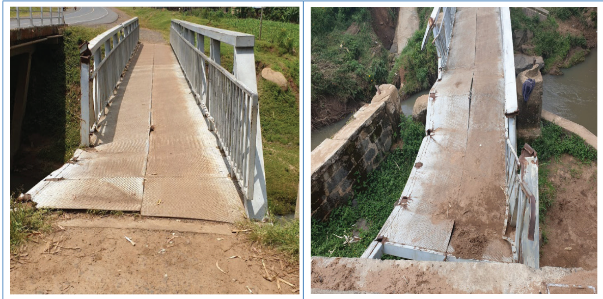
Figure 3.36 Sample photos of fracture of steel members
