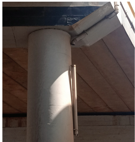
Broken drainage system
