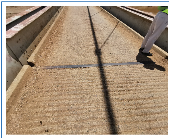
Figure 3.16 Sample photo of concrete abrasion erosion
