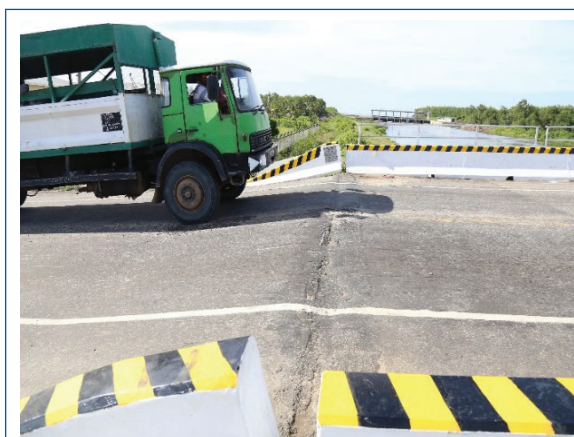
Settlement of approach slab
