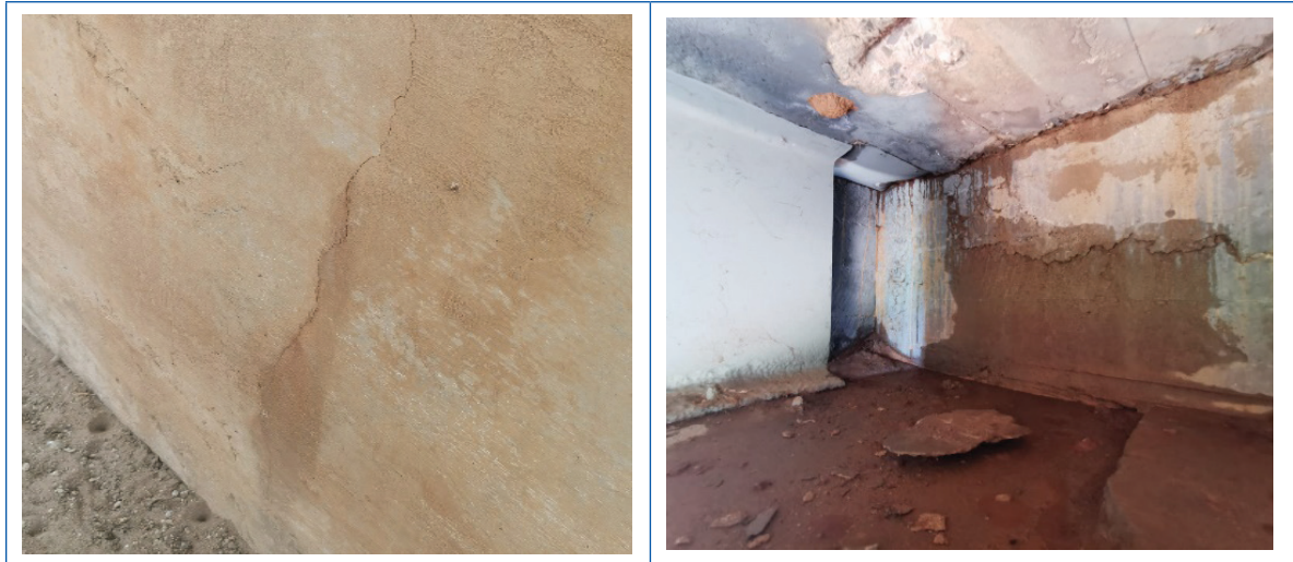
Figure 3.17 Sample photos of leakage
