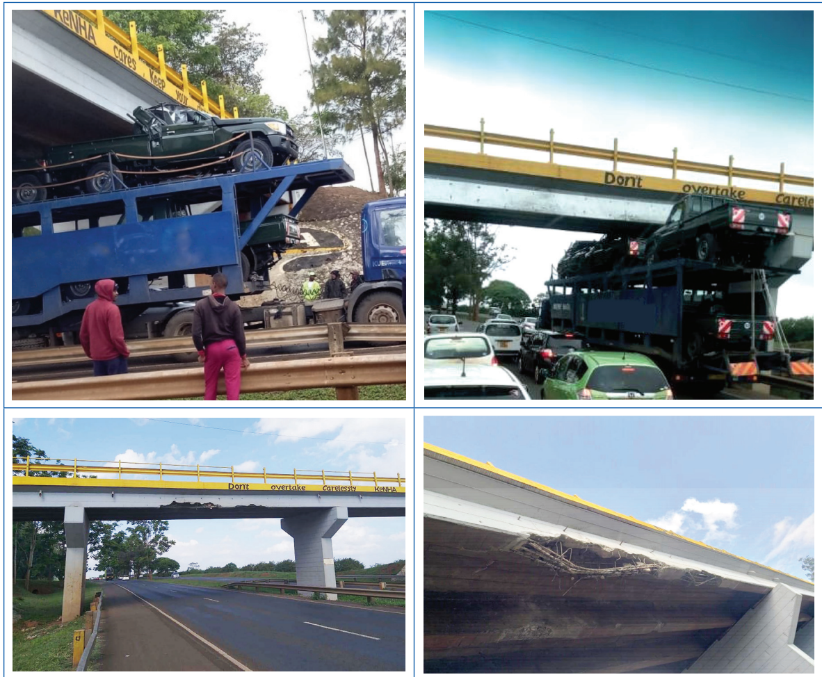
Figure 3.80 Sample photos of reinforcing members deteriorations
