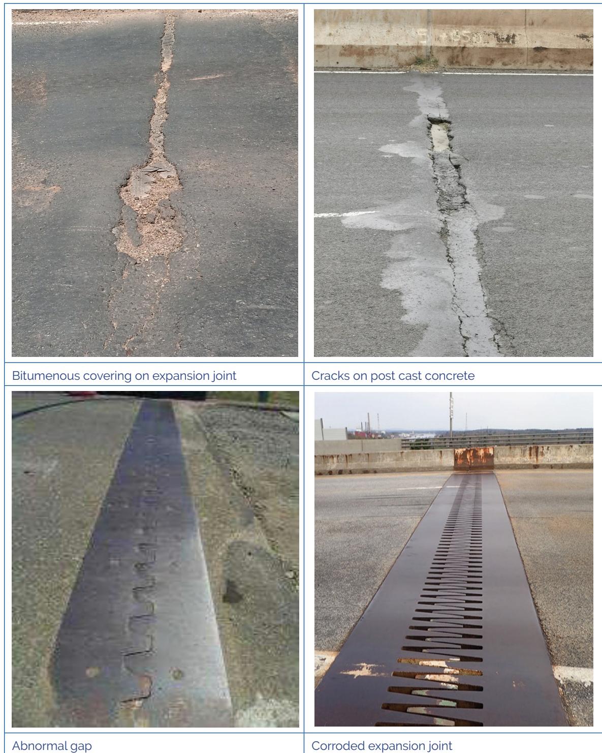
Figure 3.77 Sample photos of expansion joint deteriorations
