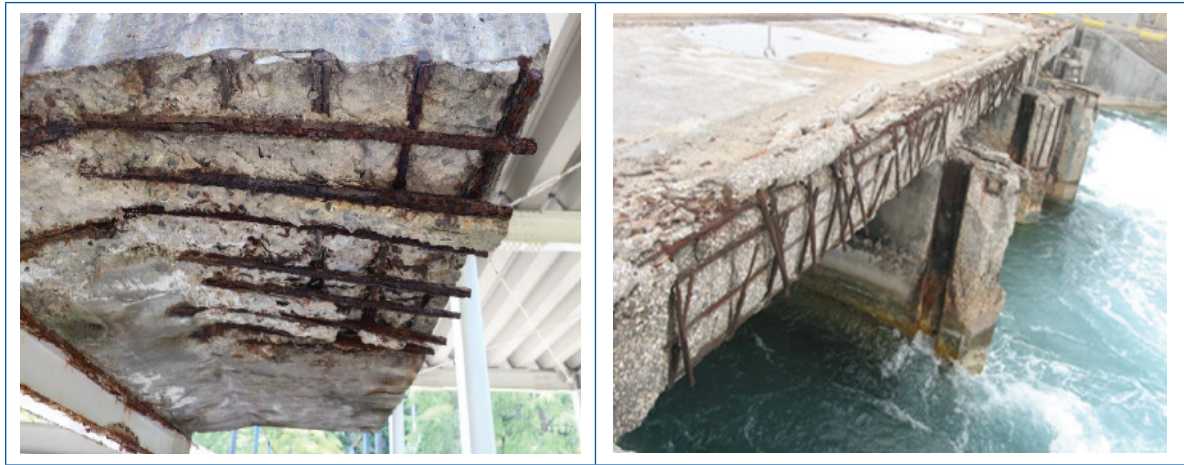
Figure 3.15 Sample photos of chloride attack
