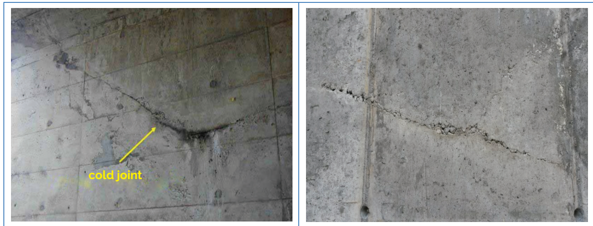
Figure 3.24 Sample photos of cold joint
