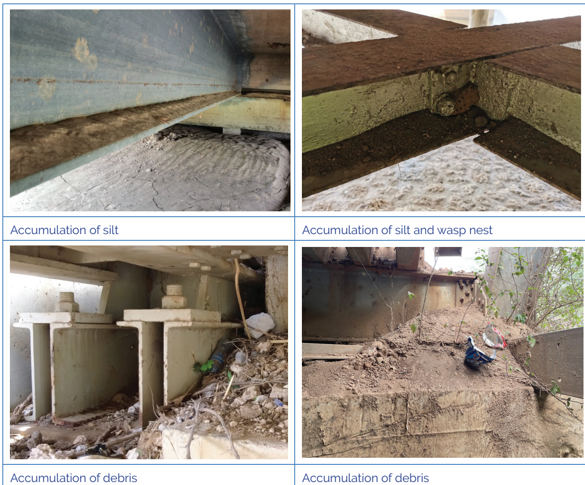
Figure 3.28 Sample photos of siltation
