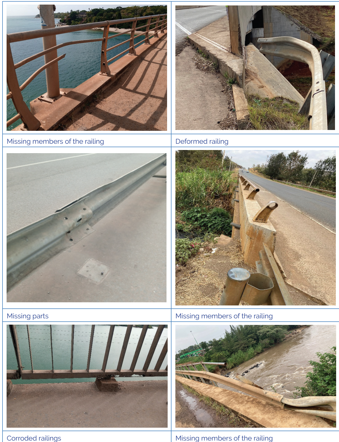
Figure 3.58 Sample photos of railing deteriorations
