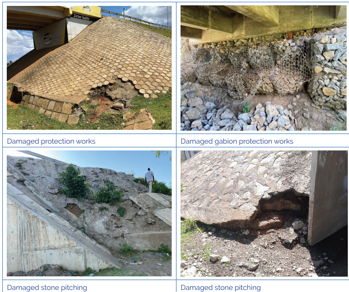
Figure 3.60 Sample photos of embankment deteriorations
