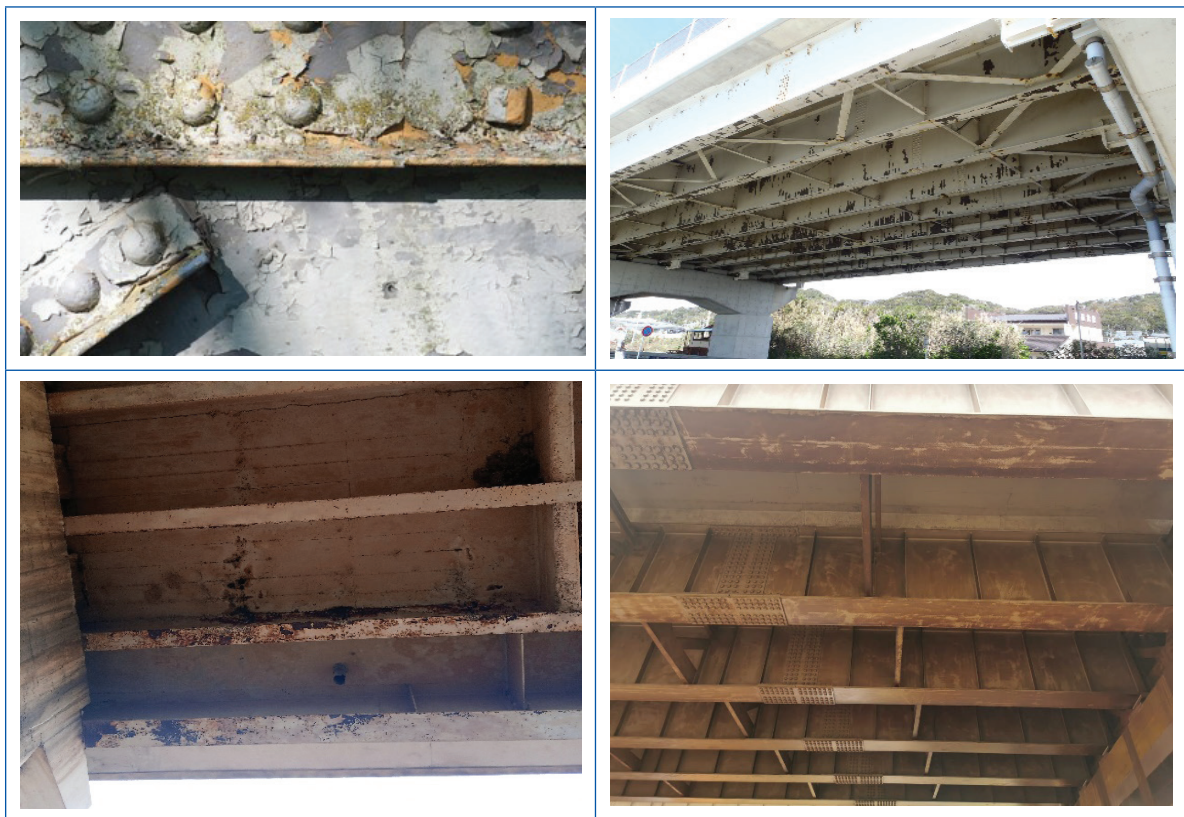
Figure 3.30 Sample photos of paint deterioration
