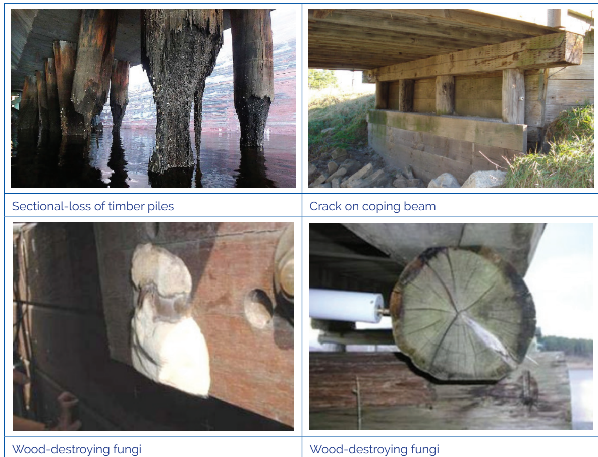
Figure 3.54 Sample photos of deterioration of timber bridge
