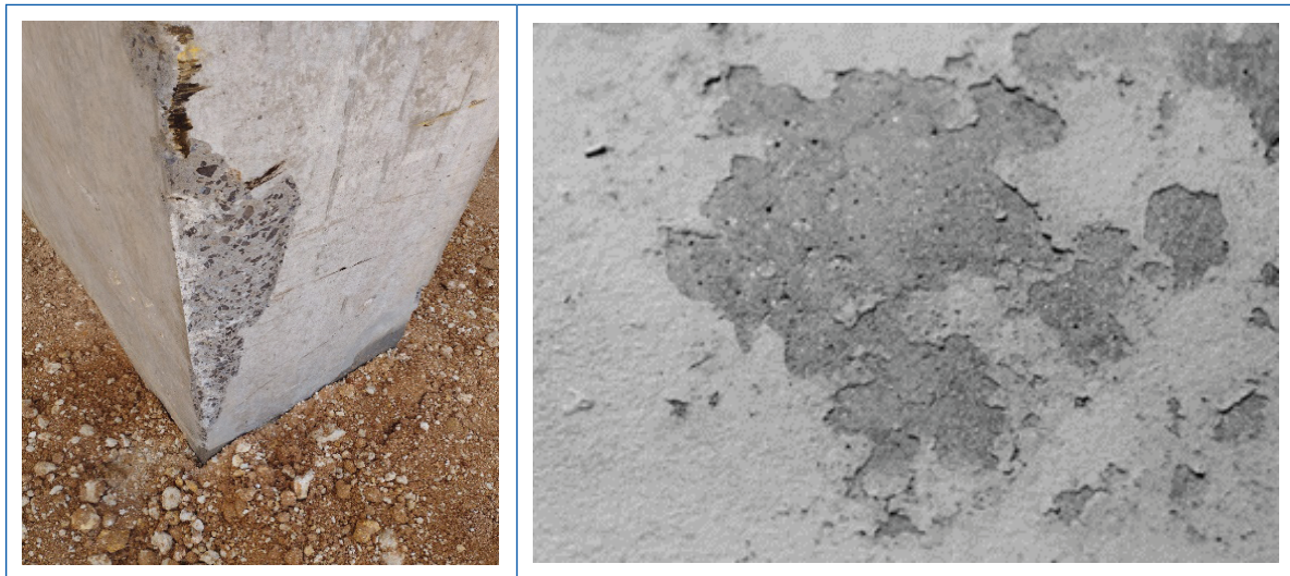
Figure 3.8 Sample photos of scaling
