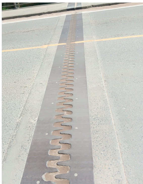
Siltation of the expansion joint
