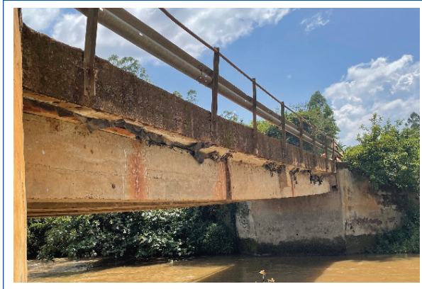
Figure 3.19 Sample photo of excessive deformation
