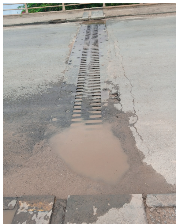
Water ponding at the expansion joint
