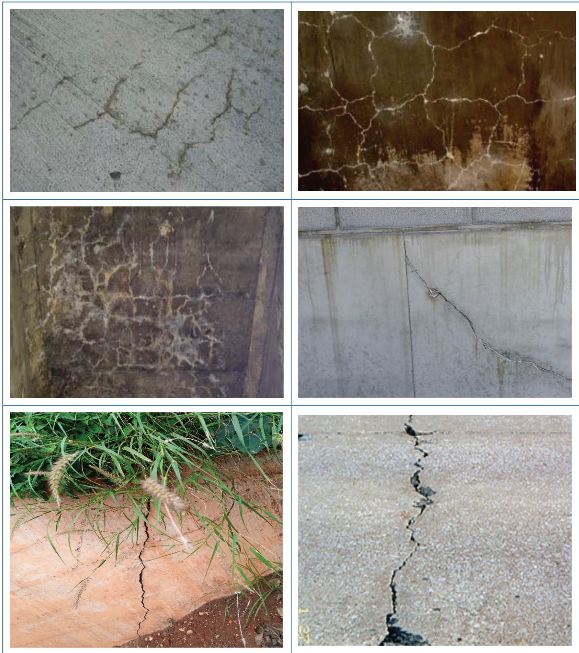
Figure 3.3 Sample photos of concrete cracks
