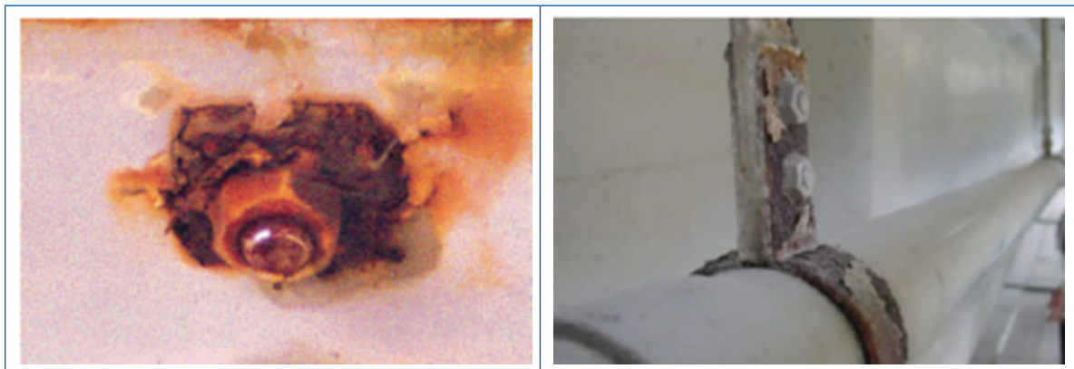
Figure 3.29 Sample photos of galvanic corrosion
