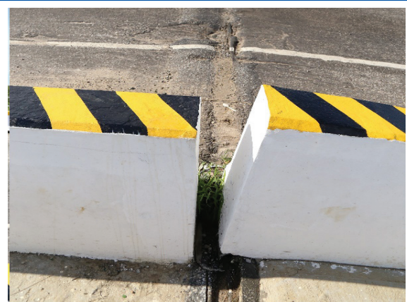
Gap at barrier end
