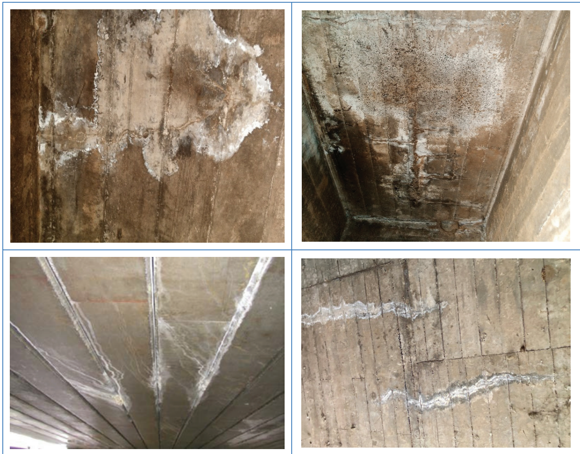
Figure 3.11 Sample photos of efflorescence
