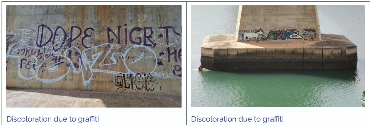
Figure 3.22 Sample photos of discoloration
