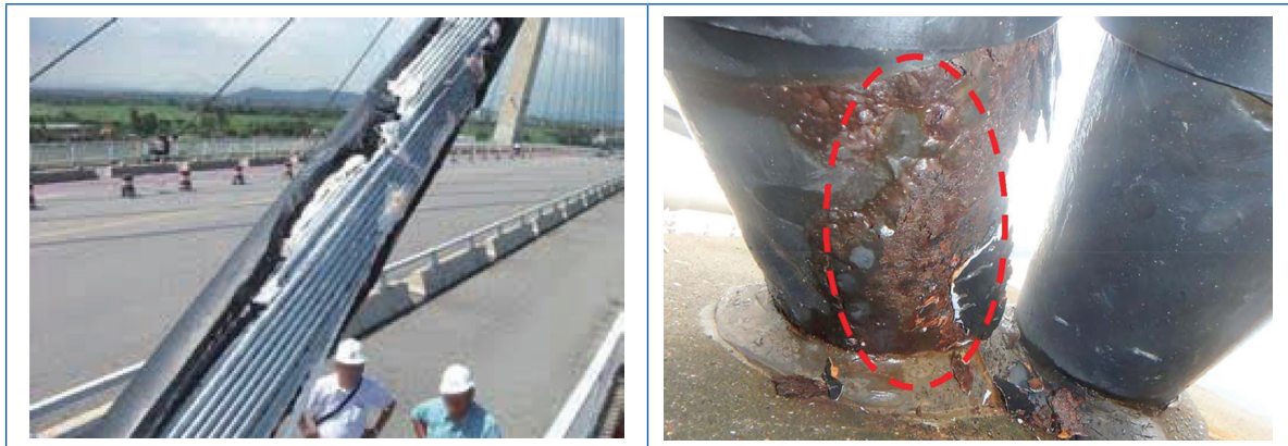
Figure 3.82 Sample photos of damage on the cable
