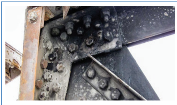
Figure 3.31 Sample photo of heat damage
