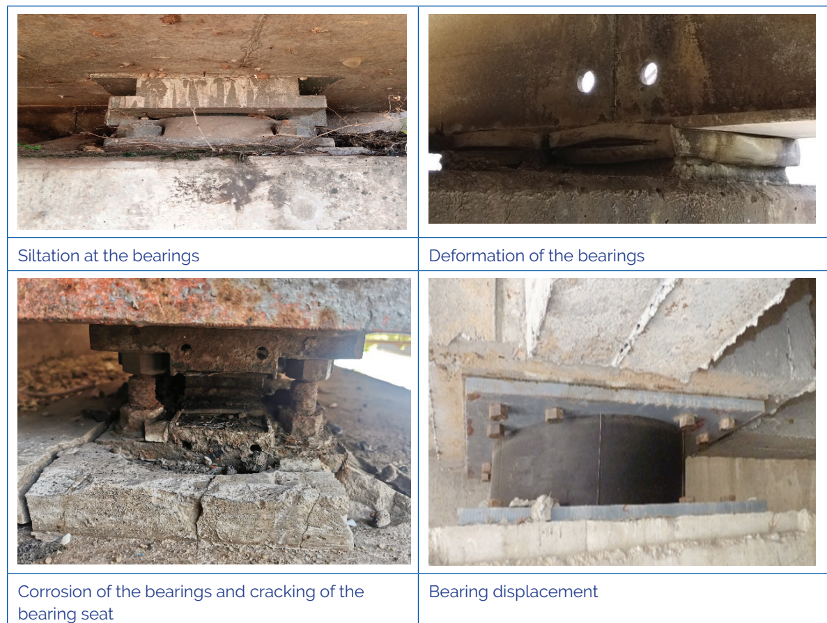
Figure 3.42 Sample photos of bearing deteriorations
