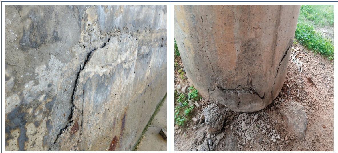
Figure 3.6 Sample photos of spalling at the pier wall
