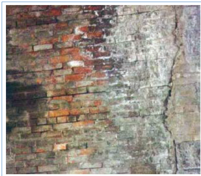
Figure 3.61 Cracks at sidewall and loss of mortar between bricks
