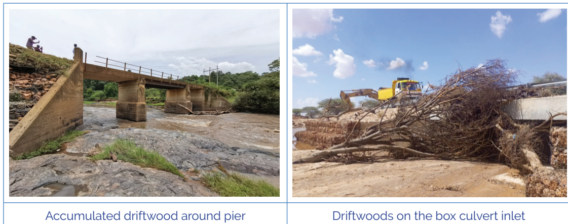
Figure 3.11 Obstructions on structure openings
