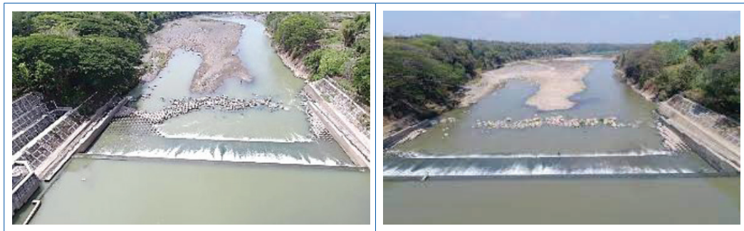
Figure 3.95 Example of progressive groundsill damage based on field observations
