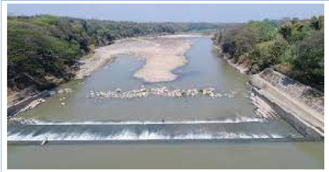
Figure 3.94 Typical damaged groundsill
